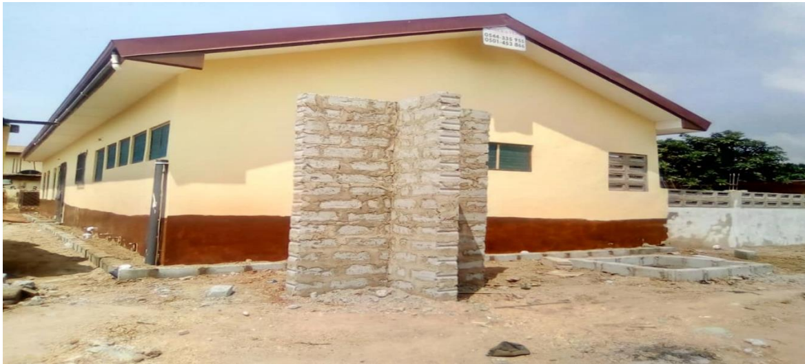
Constructed 2-unit kg block with ancillary facilities at Bubiashie 1 basic school-Okaikoi South Sub-Metro
