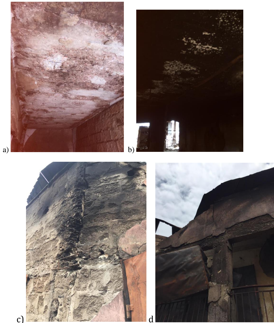
Figure 2.1 Pre-existing and Fire related Cracks
