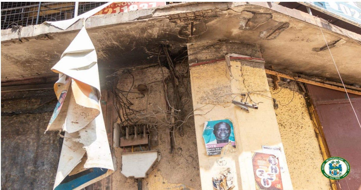
Exposed wiring on the building that caught fire captured on Tuesday 13 th July, 2021
